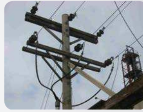
Distribution line faults
